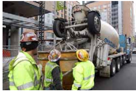
Top left: Potter and Jeremy Freeman inspect chains of crane hook. Top right: The building is constructed in close proximity to the craftsman style home in the foreground. Bottom right: Crane work on 17-story building on the Portland State University campus. Bottom middle: Bryan Ware, Jeremy Freeman, and Potter watch for crane hook to pick up the concrete bucket. Bottom left: Jason Trickett works on rebar.
