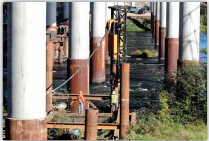
Hydraulic mechanisms at WRB use canola oil instead of petroleum-based products to reduce risk to the environment. The amount of oil it takes to cook your Holiday turkey will keep this impact hammer going for about six months. (from left) Veril Humbert and Mike Sheeley running the Hydraulic Impact Hammer while building work bridge.
